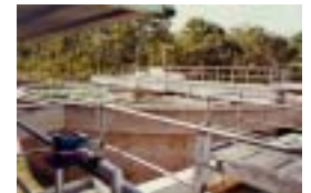
Water is treated at the water treatment plants to ensure it is safe to drink
